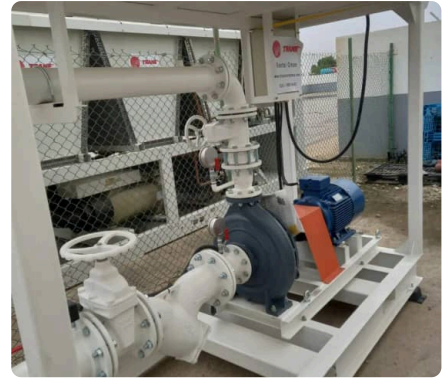
Chilled water pump skid
